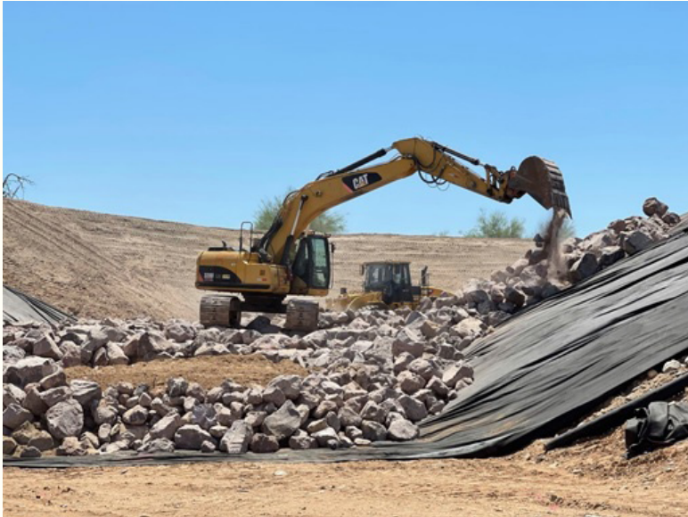
A Caterpillar 336FL excavator places large riprap designed to protect the guide banks of the new Agua Fria River Bridge.
